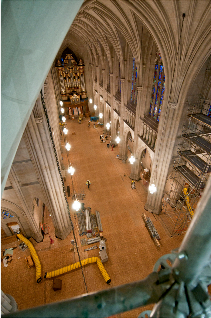
Renovation inside the nave of Duke University Chapel. Please continue to pray for the Chapel and all those working on its restoration. Photo Credit: Ray Walker, Duke Facilities architect/project manager.
